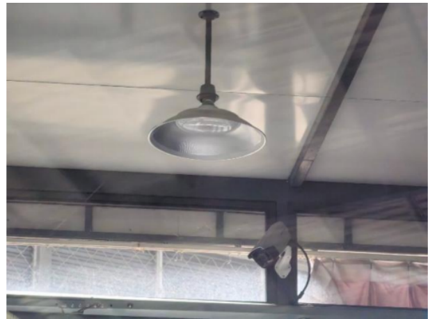
Figure 11. Sanxingdui illumination facilities
