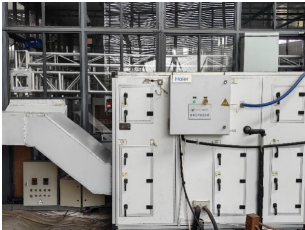
Figure 10. Sanxingdui air-conditioning system
